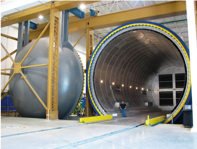
Fig. 5.6 A large autoclave that is used to make the wings of Boeing 787. An idea of the size of the autoclave can be obtained from the height of the person standing inside the autoclave. (Courtesy of ASC Process Systems Inc., Sylmar, California)
