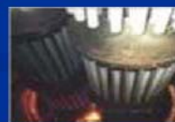
Hot gas filter system
